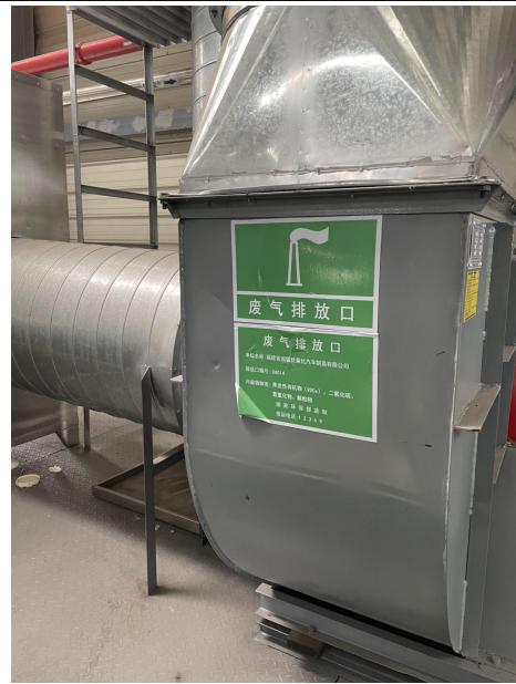
废气排放口标示
